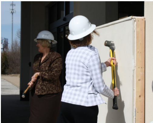
Becky Paneitz and Melba Shewmaker get the first swing in the demolition to begin the remodel of the building to become the NCPTC.
